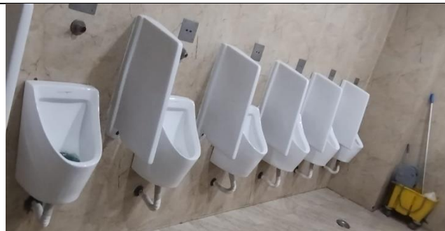
Daily Periodical Cleaning and Checking of Water Sink, Faucets, Closets to Maintain Hygiene and Prevent Water Wastage
