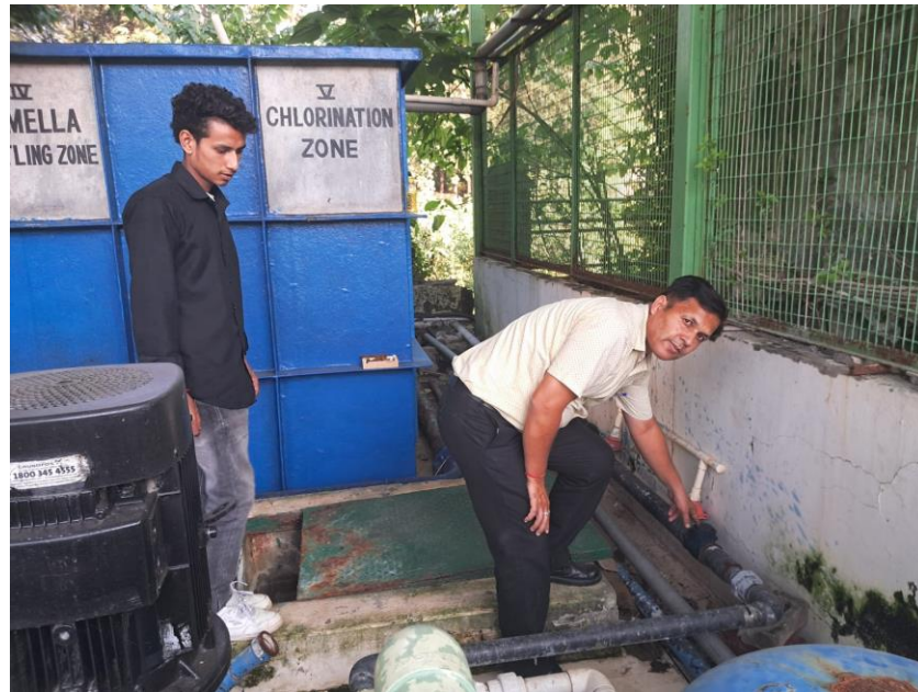
Pumps installed in STP to make treated water available for reuse in campus
