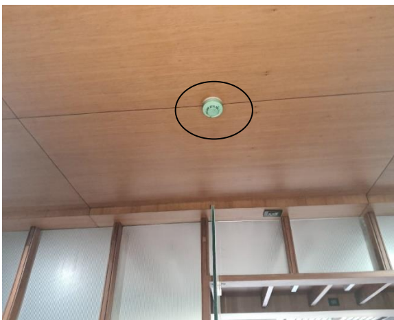
Smoke Detectors at DIT University Buildings
